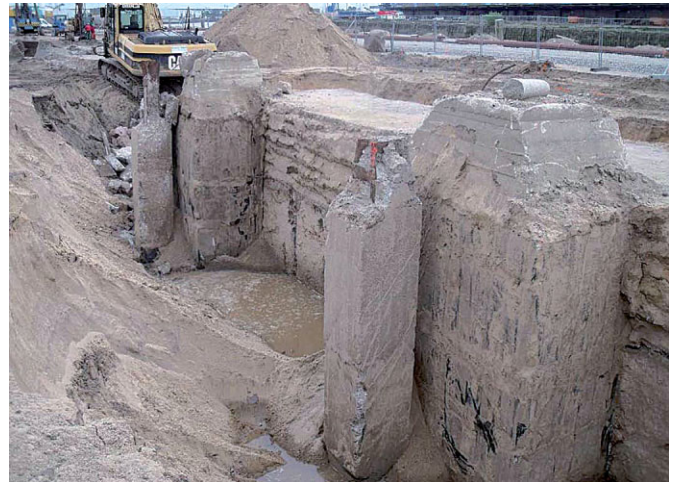
Bild 9 Hindernis Rückverankerungsblock der alten Kaimauer Obstacle presented by the tie-back anchor block of the old quay wall
